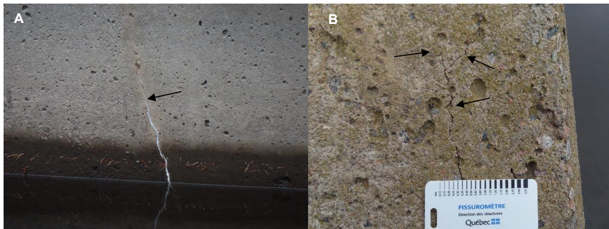
Figure 4.3: A) Vertical crack with efflorescence product. B) Longitudinal crack on the top of the wall.
