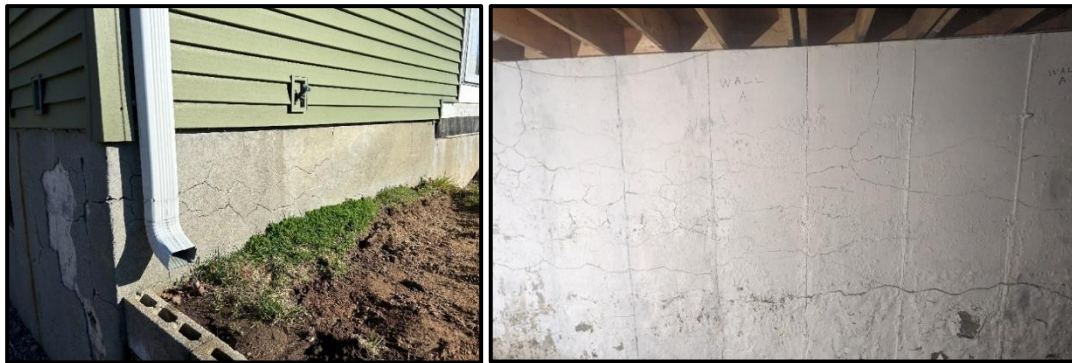
Figure 1.1: Deterioration of concrete foundation due to pyrrhotite
