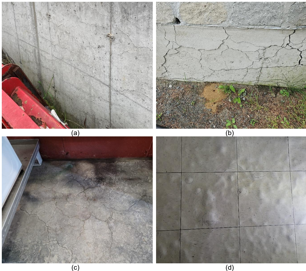
Figure 2.1: (a) Beginning of map-cracking on foundation wall; (b) Severe map-cracking on foundation wall; (c) Severe map-cracking on floor slab; (d) Blisters under vinyl covering.
