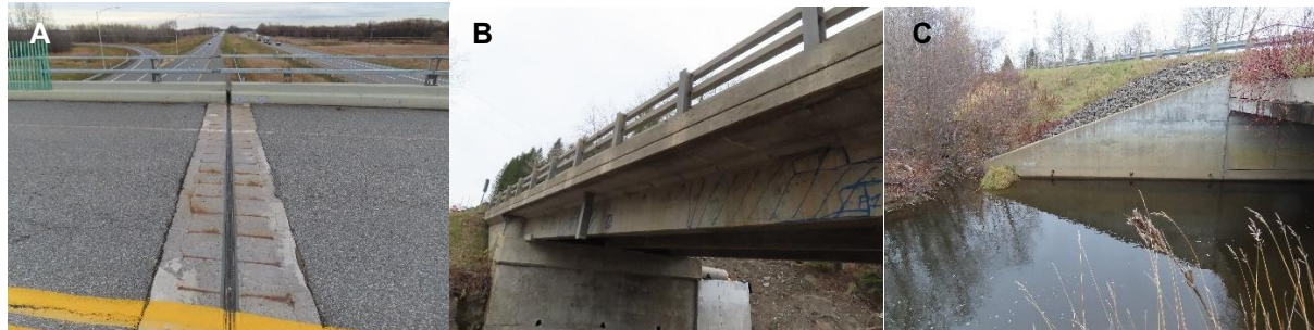
Figure 2.1: Structures with concrete containing sulfide-bearing aggregates. A) Structure 1, B) structure 2 and C) structure 3.
