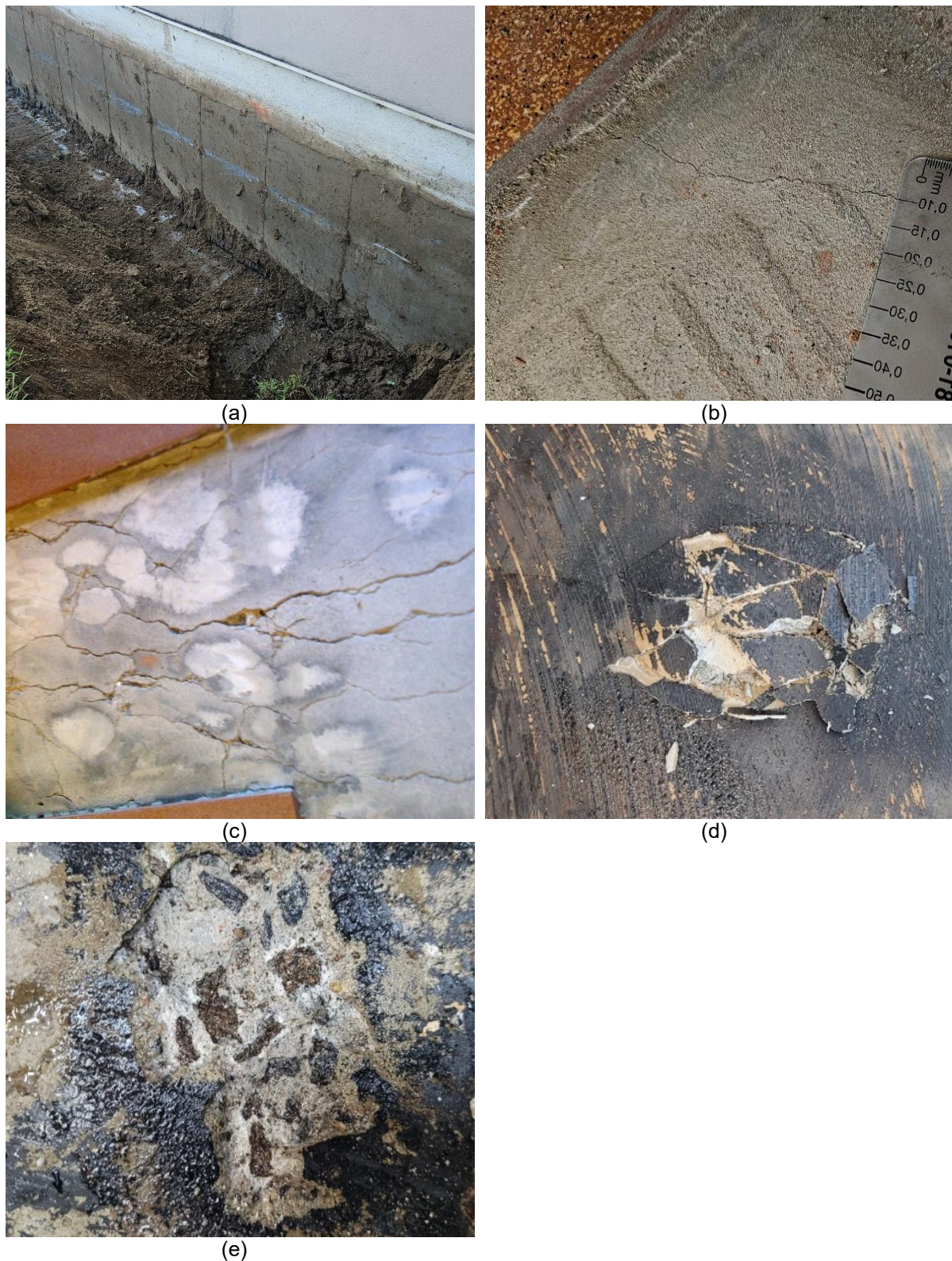
Figure 2.2: (a) Excavated foundation wall; (b) Cracking beneath ceramic tiles (internal stairwell); (c) map-cracking beneath ceramic tiles (building entrance); (d) Deformation and localized disintegration beneath vinyl covering (blister); (e) Whitish products surrounding the aggregates beneath vinyl covering (blister)
