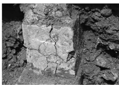
(b) Cracks at the base of the tie column
