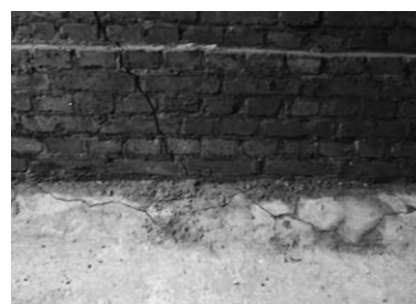
(c) Cracking in the foundation
